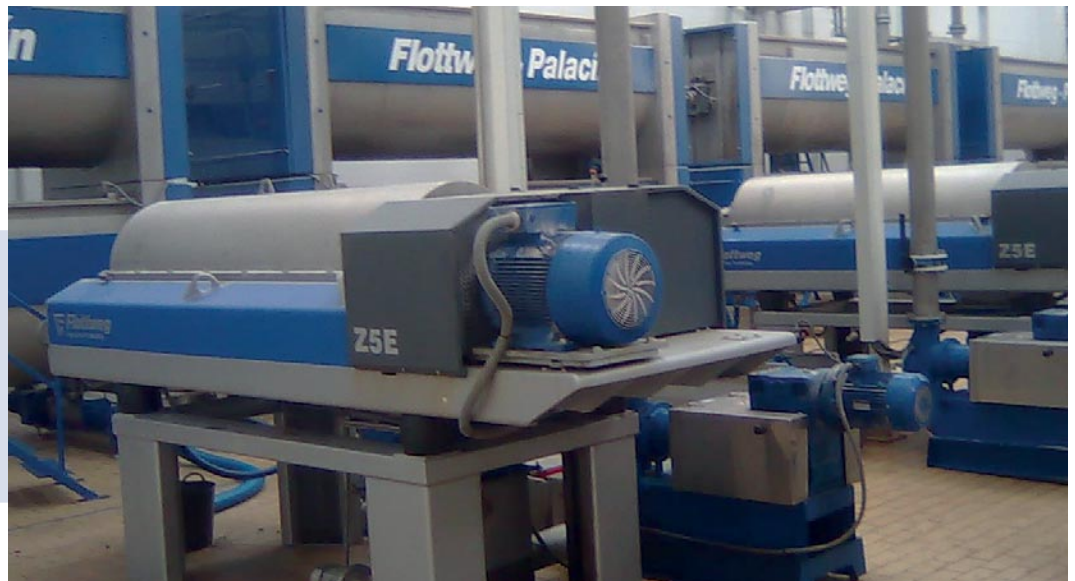
FLOTTWEG DECANTERS in a typical olive oil production plant in Spain
